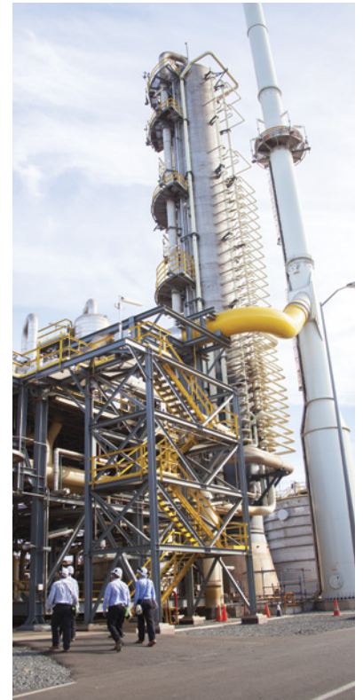
Yara Pilbara TAN Plant
