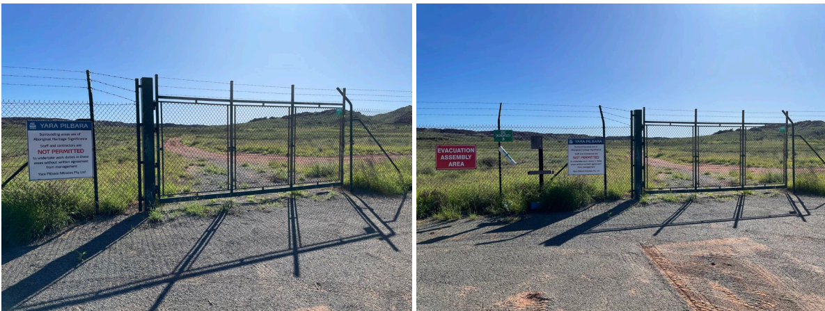
Condition 8: 2.5 m chain link perimeter fence and signage near northern perimeter emergency exit (east side)
