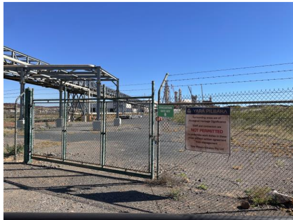
Condition 8: 2.5 m chain link perimeter fence and signage near western perimeter emergency exit (north side)- replaced with spare (05/07/2023)
